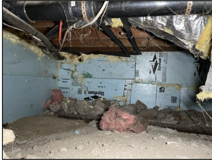
Exposed combustible insulation
