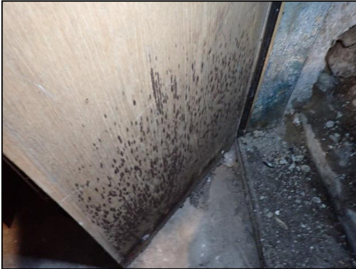
Moisture damage at bottom of door
