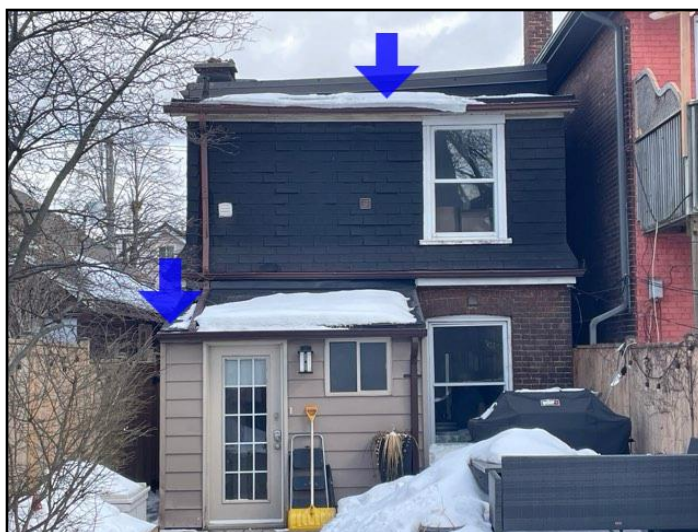
Improper slope, ponding
