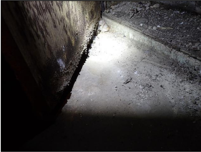
Moisture damage at bottom of door
