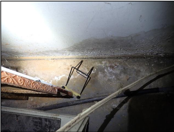
Water stains (inside)
