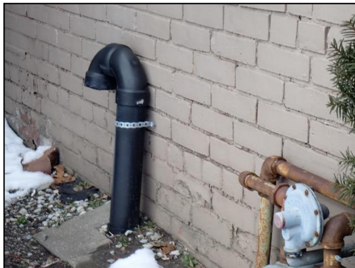
Suspected waste vent
