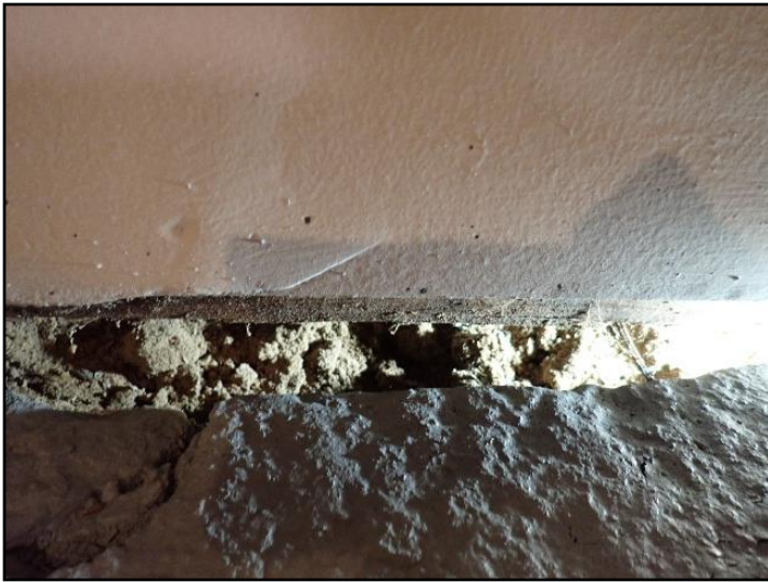
Gap in slab
