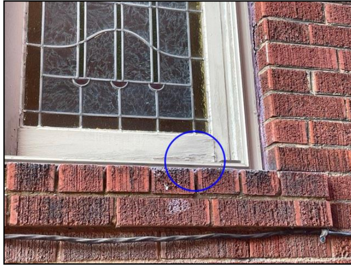
Regular maintenance needed
