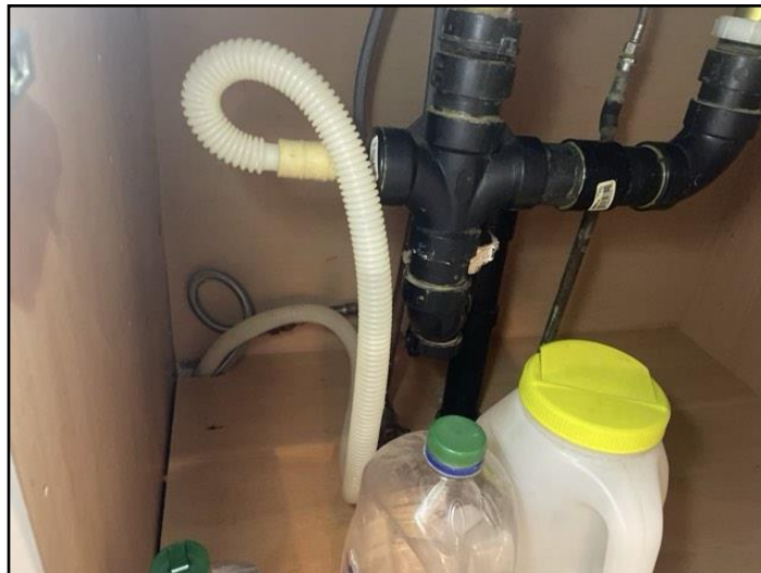
Backflow prevention high loop missing
