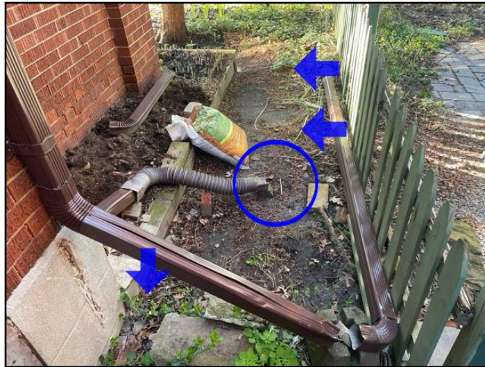
Discharge too close to building
