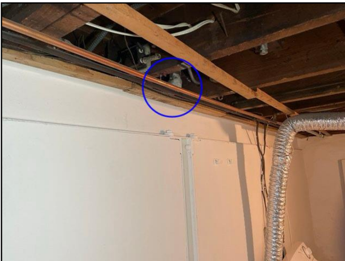
Insulation on boiler piping
