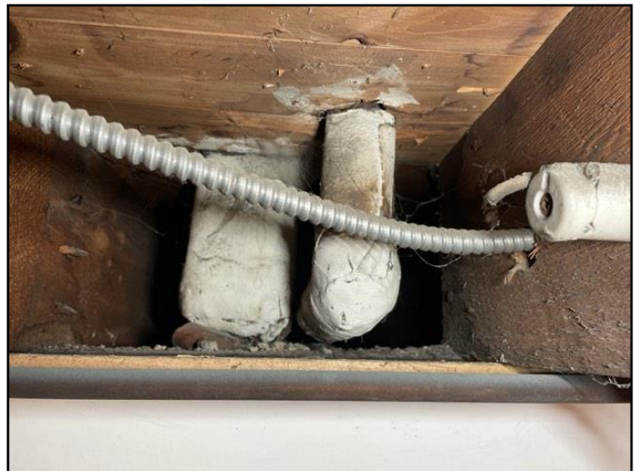
Insulation on boiler piping
