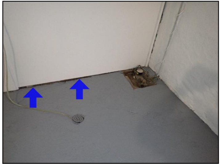
Gap in slab / beneath wall
