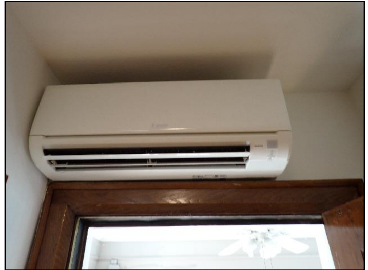
Indoor unit - Above main floor entry
