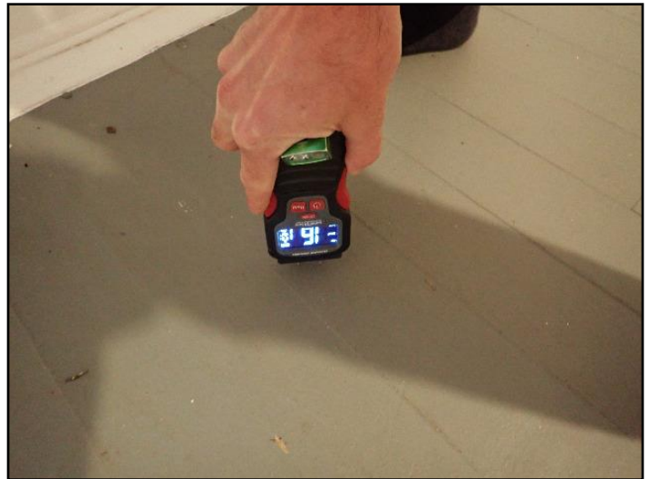
Elevated moisture - floor
