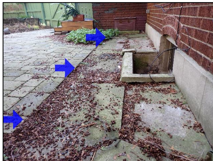
Improper slope or drainage
