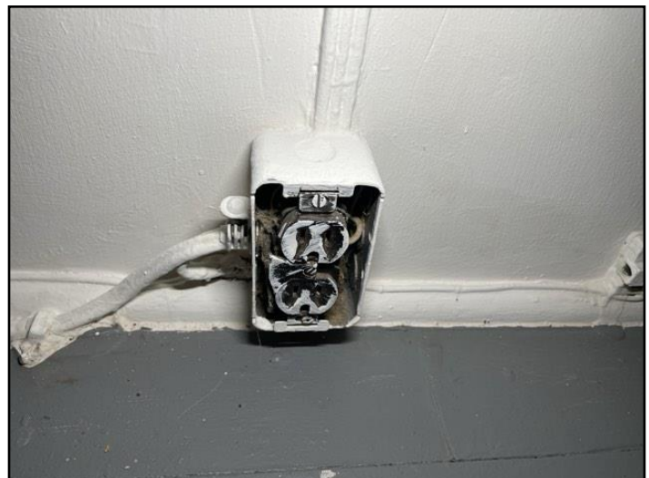
Missing cover plate
