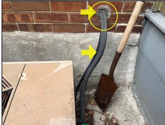
Insulation - missing; Poor Seal at Building
