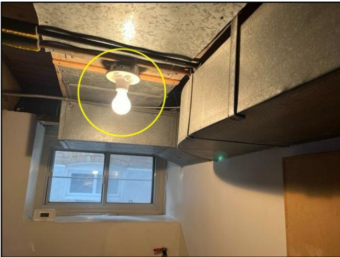
Exposed bulbs: Example, Rear Basement
