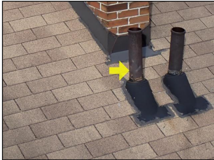
Cast iron waste stack
