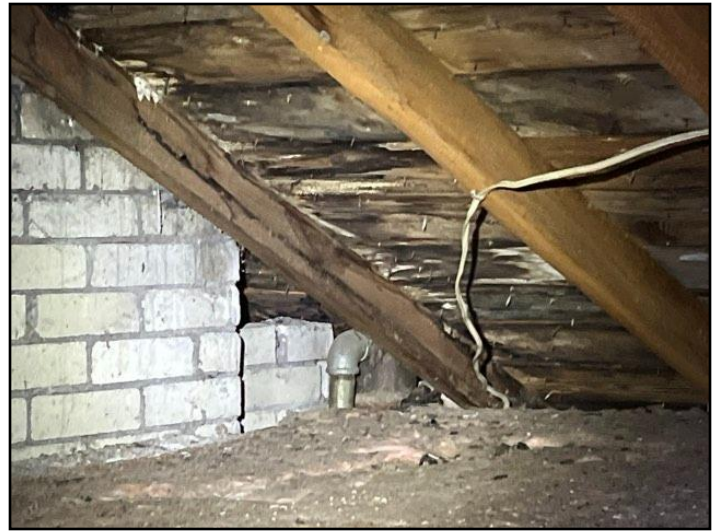
Detail: Water stains
