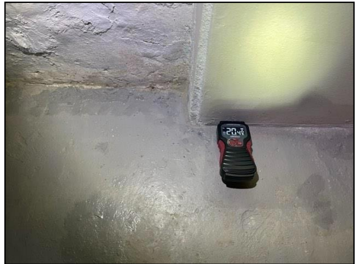
Evidence of moisture noted: Rear Left
