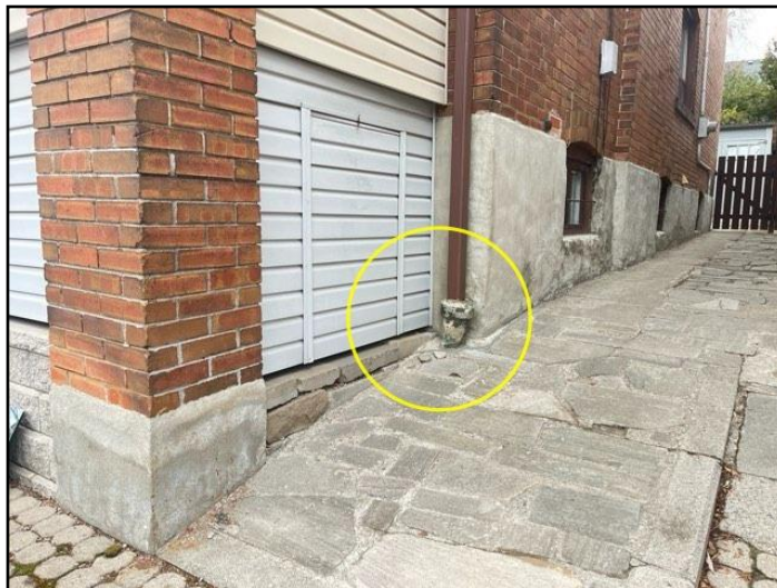
Discharge below grade - See Exemption in Appx
