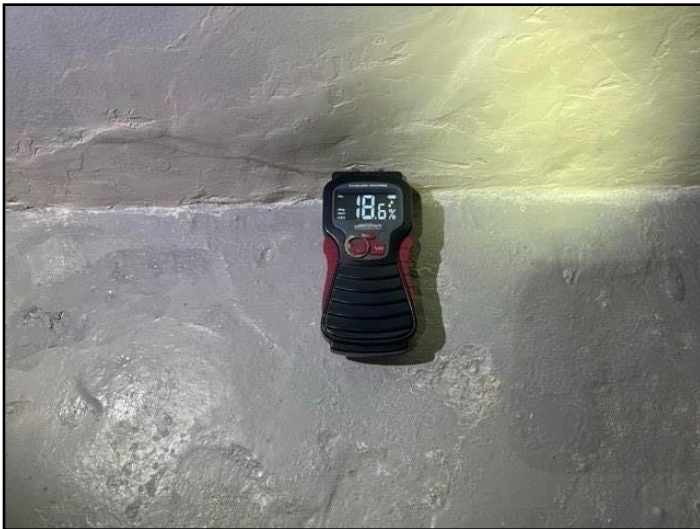
Evidence of moisture noted: Rear Middle
