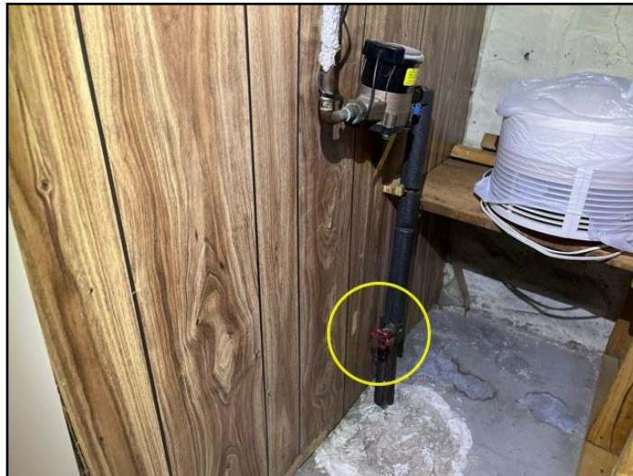
Main Water Shut-off
