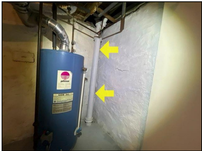
Cast iron waste stack
