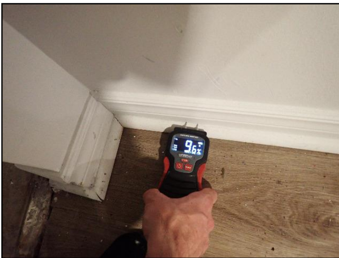
Front - Typical reading noted - Dry
