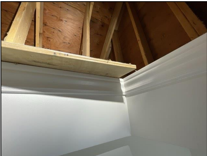
Not insulated and not weatherstripped
